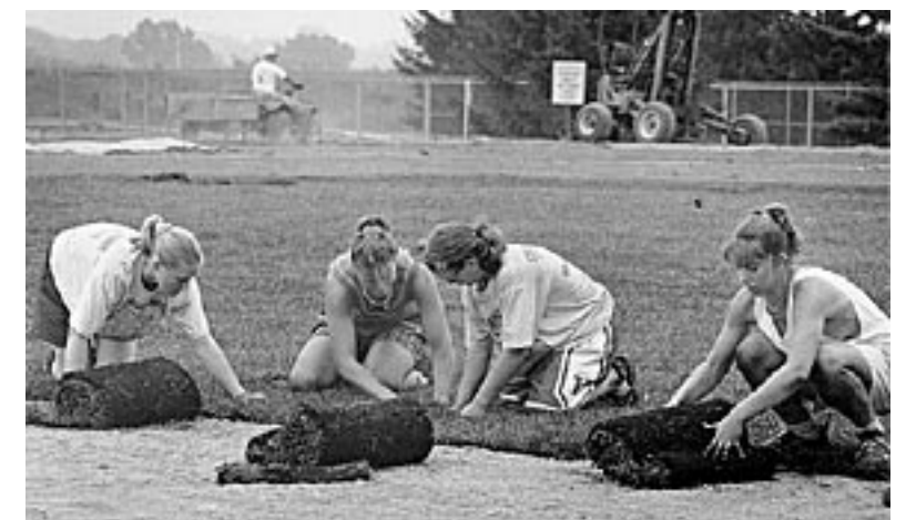
Getting the new stadium built and the field sodded was just another good team effort.
